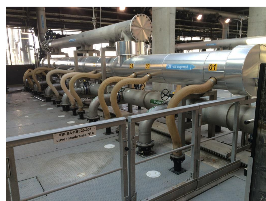
Fig 3. Filtration zone of studied full-scale MBR
